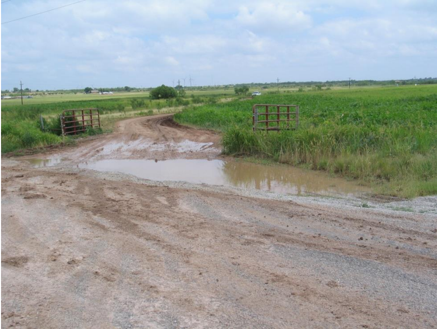
Drainage problem at driveway
