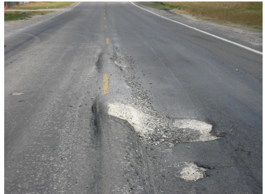
Pavement shoving, loss of surface
