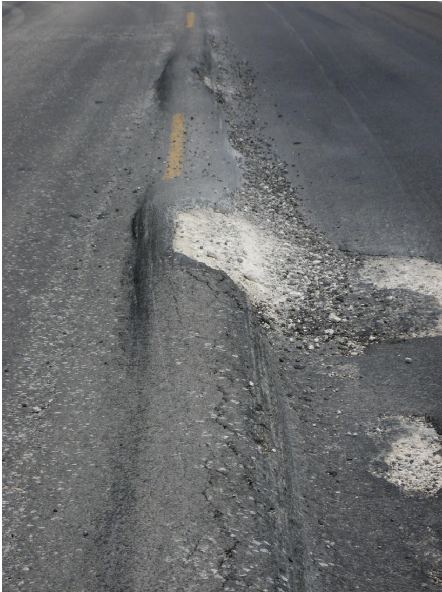
Pavement shoving, loss of surface
